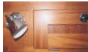
Light fixtures are steel rather than plastic.
